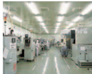
Exposed Fluorescent Lights
