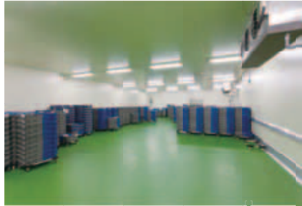
Shipping preparation room (Refrigerating room)
